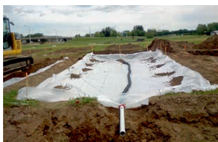
Fig. 1: Excavated plot with the two plastic sheets and the drain used to collect leachate.
